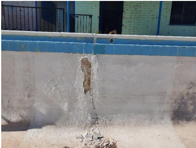
Lap pool expansion joint – significant structural failure, caulk and plaster failures.
