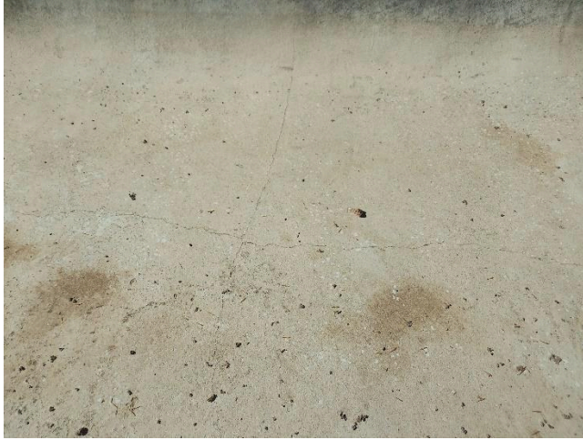
Significant cracks in Lap pool floor.
