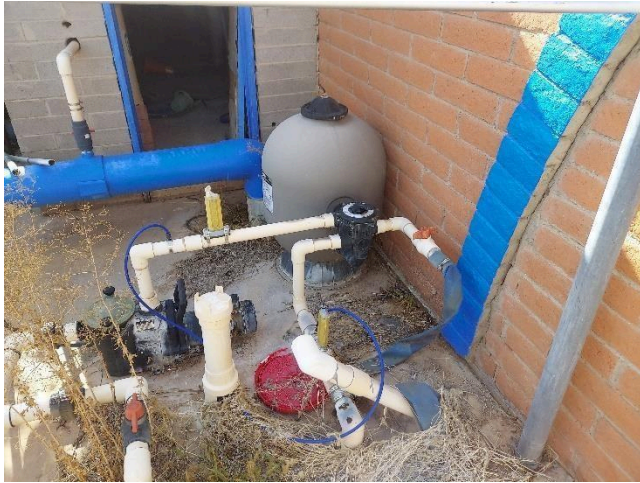
Wading pool filter plant – backwash does not tie into sanitary sewer, flow meters not located per manufacturers recommendations.
