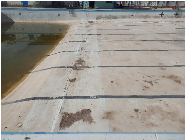
Lap pool expansion joint – failed caulk across entire joint.
