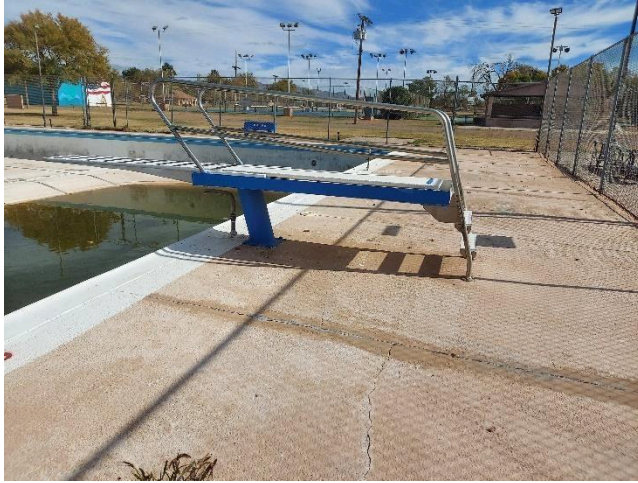
Significant cracks in deck. Minor corrosion on diving tower.
