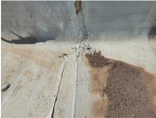
Significant structural crack in Lap pool wall translating through tile bands.
