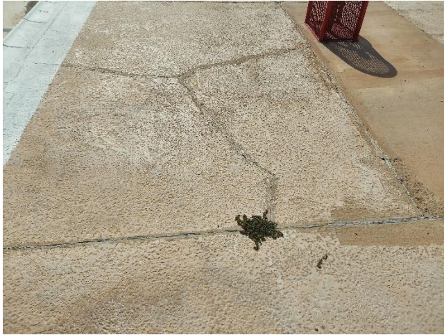
Significant cracks in deck with some separation. Failed caulk in joints.
