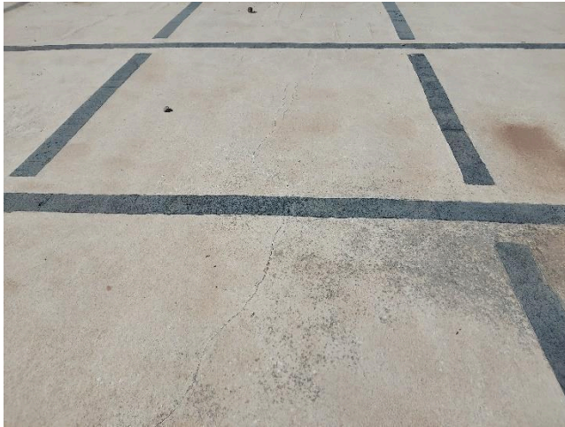
Lap pool floor – structural failure and separation with flexure cracks.
